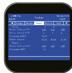
UPS Cabinet Control Panel
